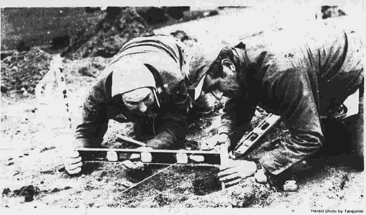
Veterans' memorial work under way Tom Flaherty, left, and Ottavio Forlino, both of the Andrew Ansaldo Co., mark off Tuesday what will be a sidewalk at the Vietnam Veterans Memorial Park. The Manchester-based Ansaldo construction firm has started initial work at the half-acre site at Main and Center streets. Initial site work includes installing water and electric lines, and building sidewalks and a concrete base for a monument. The committee planning the park is hoping the park will be ready for dedication by Memorial Day.
